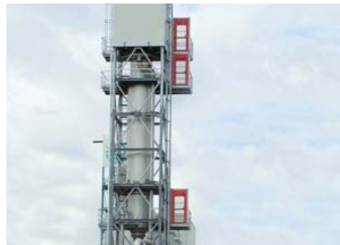
Drop pelletizing tower of a DROPPO® 300 system for chemicals
